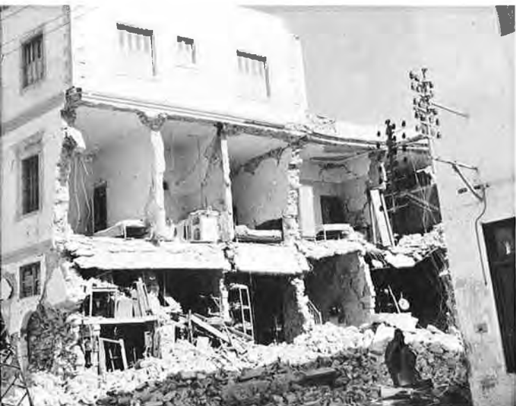
Fig. 20. Typical Failure of Masonry Construction, Talborjt District
