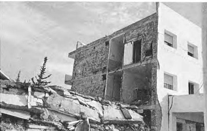
Fig. 28. Close-up of Collapse; Note Lack of Connection to Adjacent Structure
