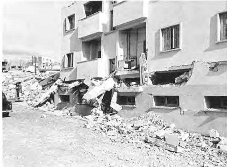
Fig. 24. Complete Collapse of First Story of Building Shown in Fig. 22
