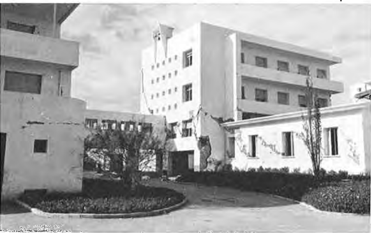
Fig. 25. General View of Lyautey Hospital; Note Diagonal Cracks in Masonry
