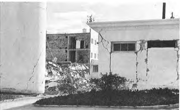
Fig. 27. Collapsed Maternity Wing, Lyautey Hospital
