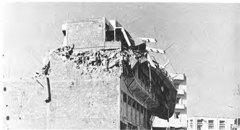
Fig. 50. Sud Building from the Southwest, Note How Third Story Has Collapsed Toward the Right (SE)
