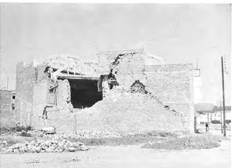
Fig. 37. Roof System of Rialto Theater Damaged by Collapse of Masonry Bearing Wall
