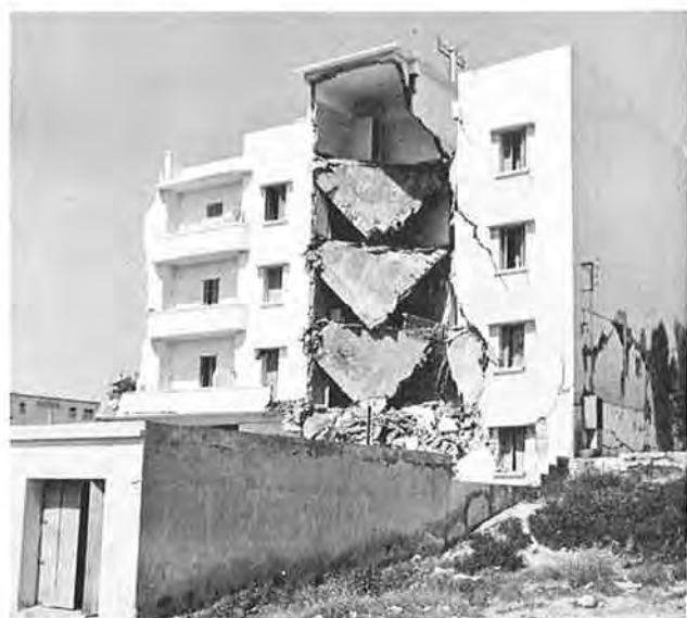
Fig. 33. Collapse of Masonry Bearing Wall Leaves Floor Slabs Unsupported
